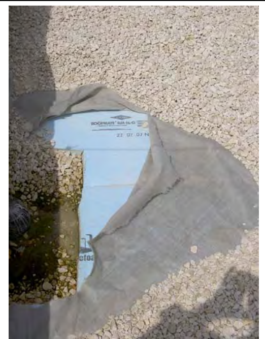
Thermal Insulation of roof
