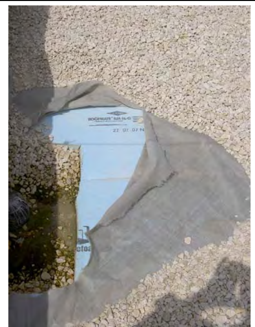
Thermal Insulation of roof
